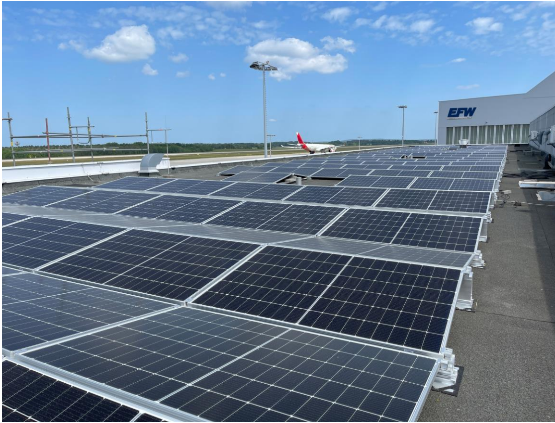
Solar Panels at EFW's facility in Dresden, Germany.
