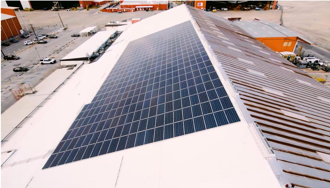
Solar panels installed atop one of the facilities at San Antonio Aerospace, U.S.
