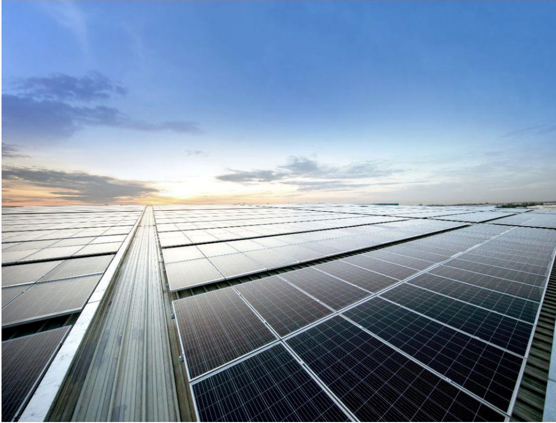
Solar panels installed atop our hangar facilities in Singapore
